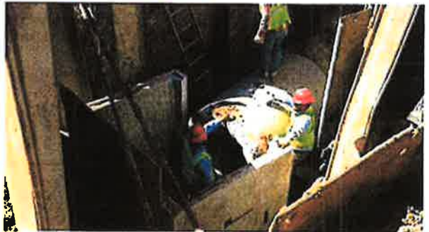
Installing 48-inch storm sewer connection between the Town & Country Blvd. and Town & Country Way storm water box culverts
