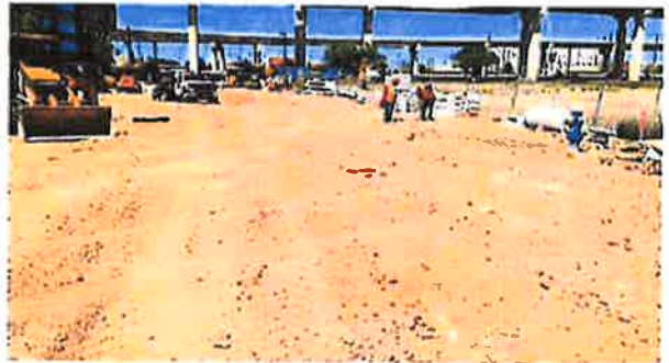
Town & Country Blvd. pavement subgrade stabilization and layout work in progress—looking north
